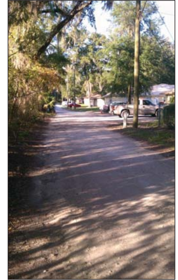
This photograph was taken looking North on NE 57th Ave., from intersection at NE 32nd St. This documents the dirt roads in residential areas of the Study Area. There is no stormwater infrastructure in place to mitigate ponding and flooding.
