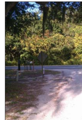
The photograph to the left exhibits deteriorating infrastructure/pavement. This photograph was taken at NE 64th Ave. Rd. at Route 326. Stormwater runoff has etched a path of flow from the pavement, resulting in cracking and deterioration of the pavement.
