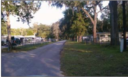
Photographed while looking East on NE 32nd St. at the intersection with NE 56th Ave. This stretch of pavement fails to include curbs, gutters, sidewalks, or any form of stormwater infrastructure. The pavement is crumbling on the edges.
