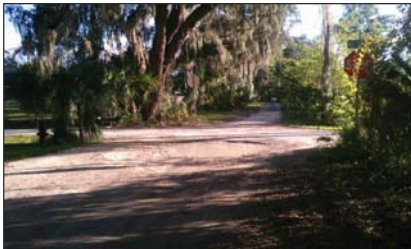
Photographed at the Intersection of NE 57nd Ave. and NE 32nd St. This is a dirt road in a residential area. As a result of the lack of pavement, severe ponding has occurred in the middle of the dirt road adjacent to the stop sign.
