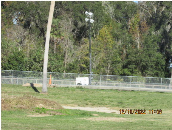
Portable stadium light with generator.
