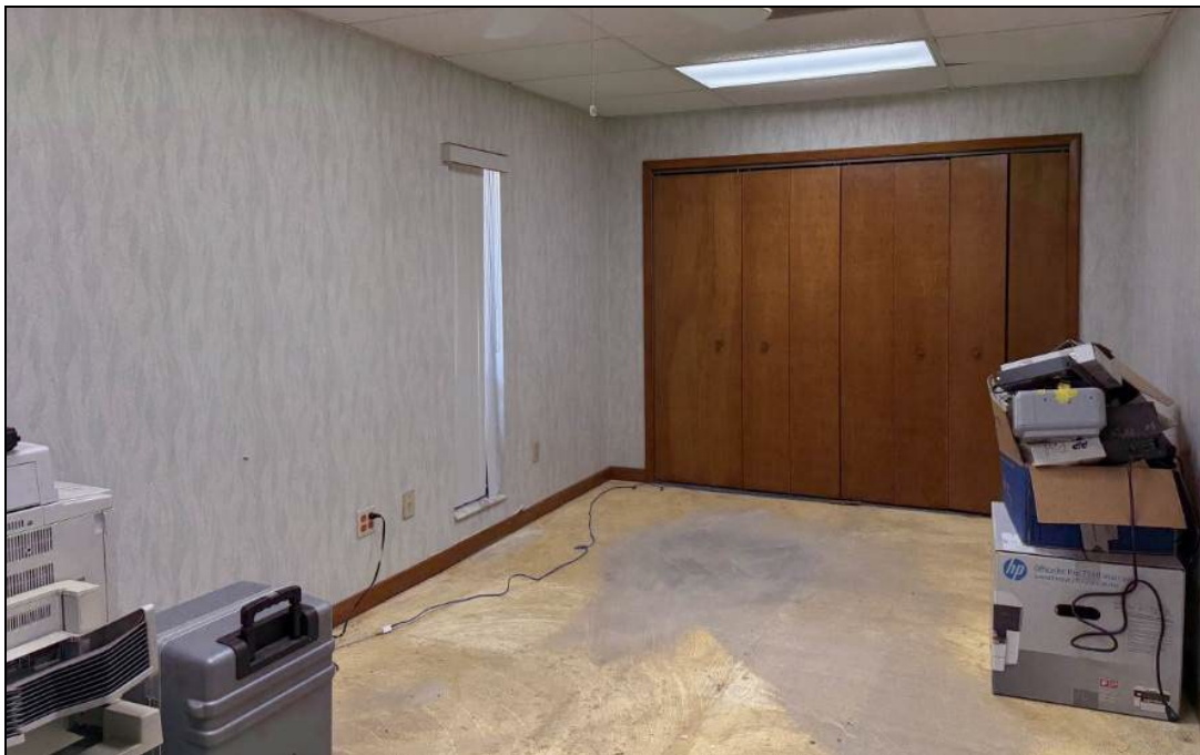
Typical office space in the building; note that floor coverings have been removed in order to accommodate installation of new carpeting.
