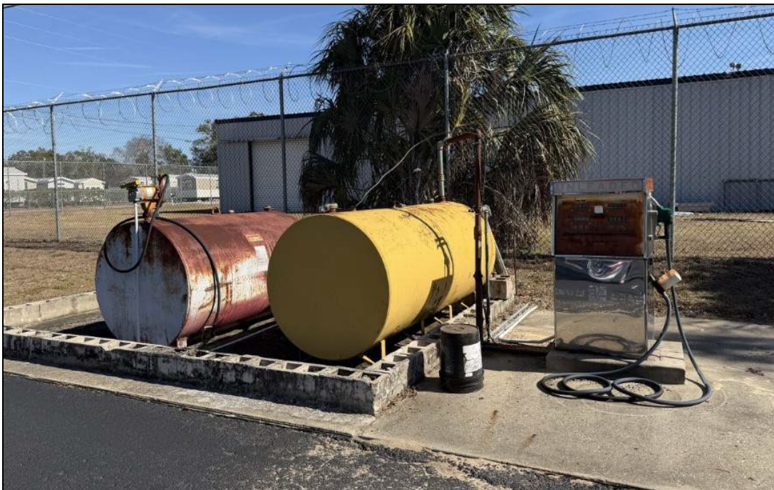
Close-up view of the fueling station on the site, which includes a concrete pad, a fuel pump and dispenser, and two 500-gallon above-ground fuel storage tanks.
