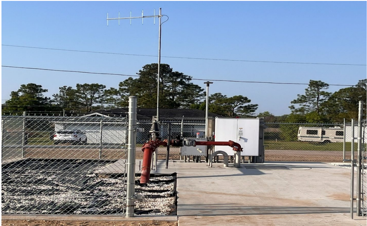
Figure 2. Lift Station no. 51
