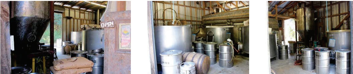
8. Views of new building area to the east/left of the original distillery structure.
